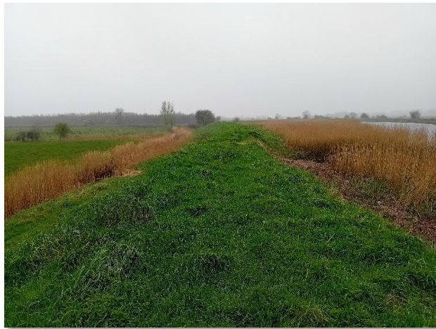
Image 4-11: E9 – improved grassland on embankment footprint fringed by wet grassland and reed and large sedge swamp
