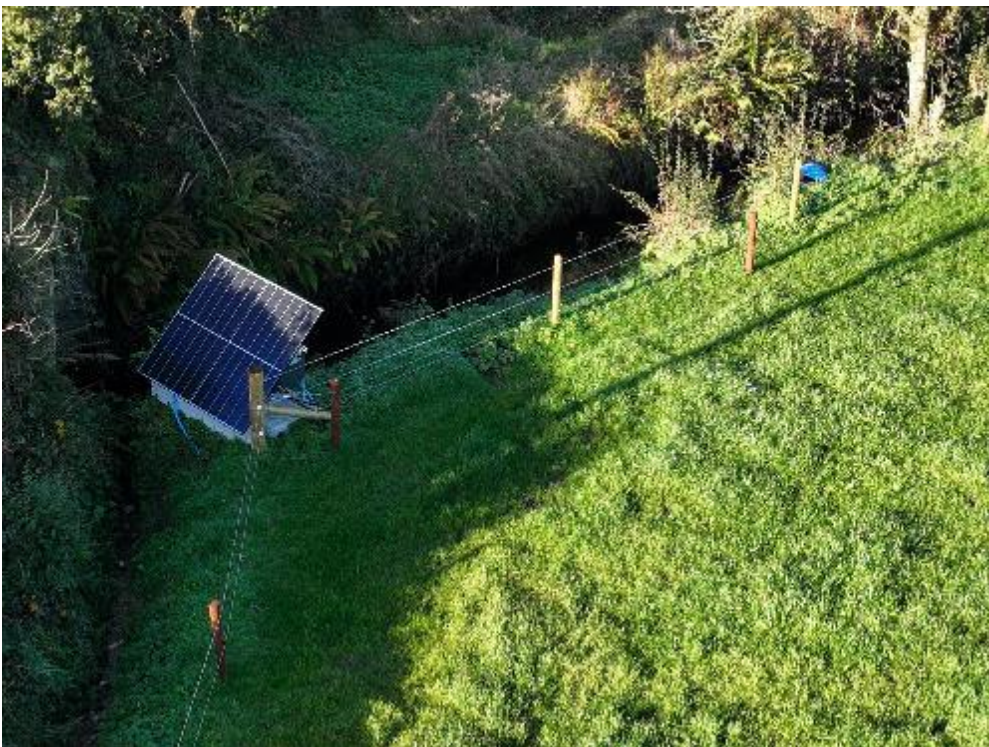
Plate 2: Aerial view of fencing and solar pump on the Mountnugent River
