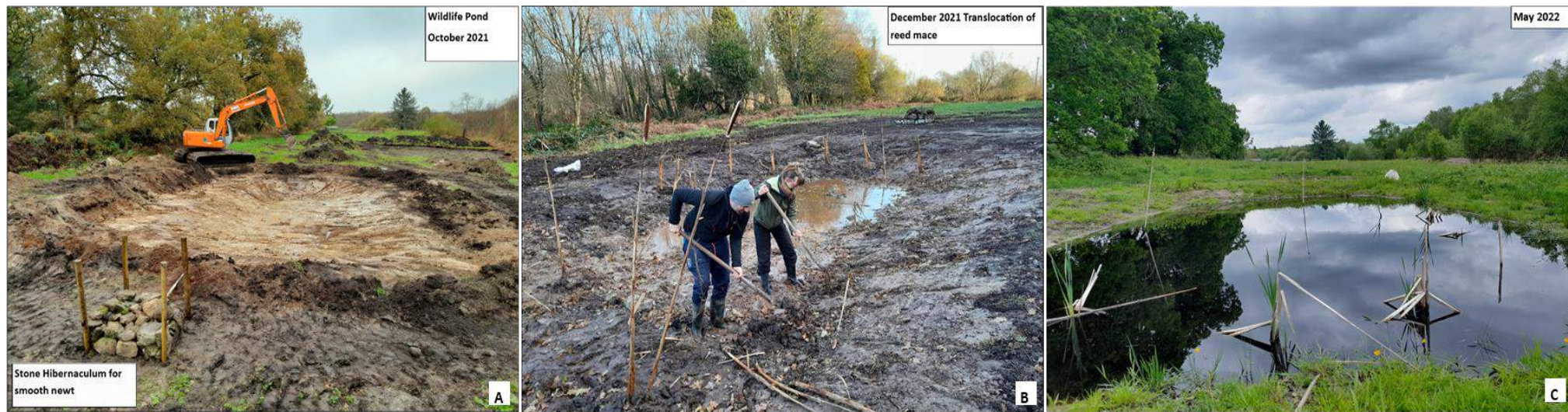
Plates 4.3 (a) (b) and (c): The pond was excavated in agricultural grassland in October and November 2021 and a stone hibernaculum (micro-habitat) for amphibians was created (A); reed mace was translocated from a donor site to the pond margins in December 2021 (B); and the successful establishment of reed mace in May 2022 (C).
