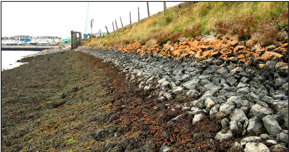
Plate 2: View of distinct vertical zonation pattern along Malahide railway embankment – outer (eastern) face.
