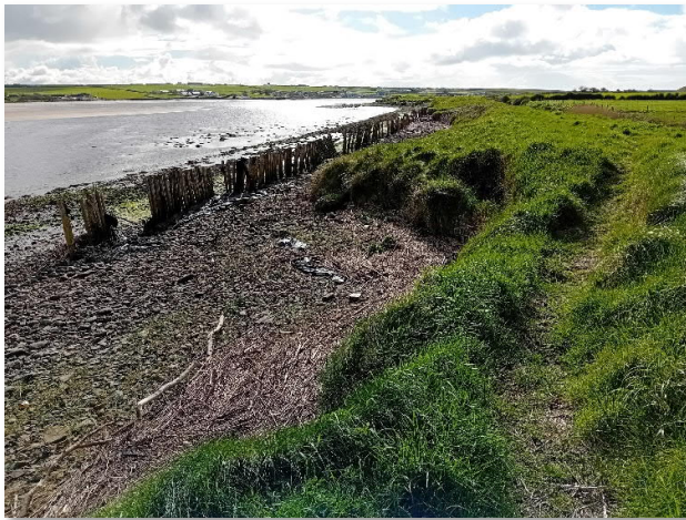
Image 4-1: Footprint of eroded embankment looking west
