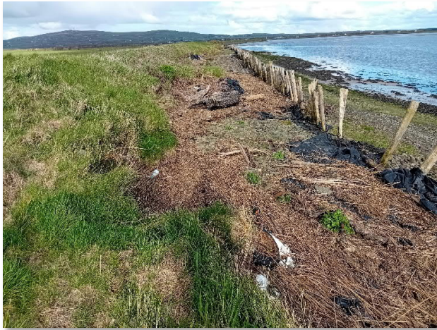
Figure 4-5: Eroded embankment looking east
